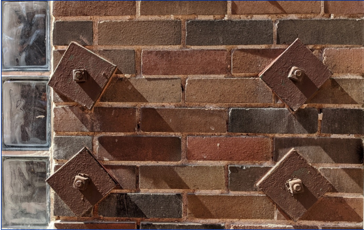
Figure 19: View of rusted metal brackets on northeast elevation
