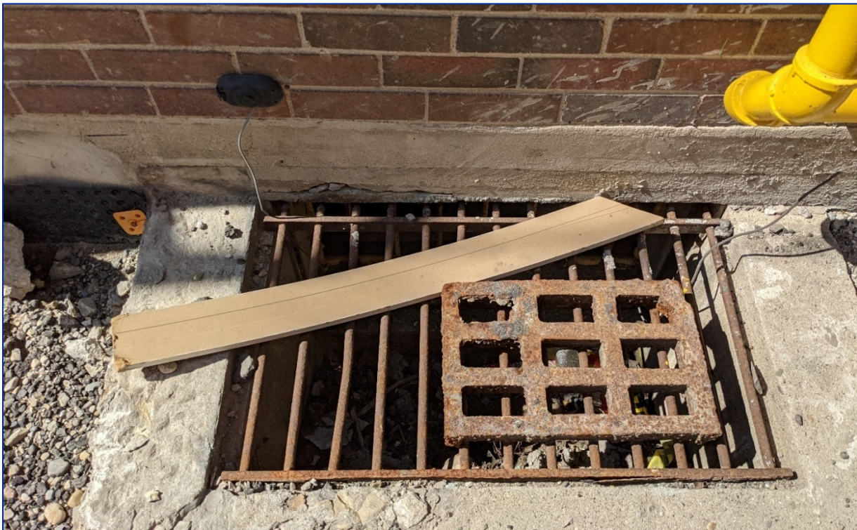
Figure 20: View of rusted metal grate on northeast elevation
